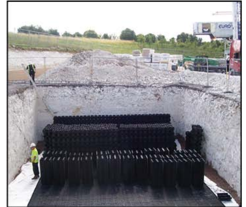
Above: One of the larger tank installations
